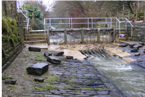
Plate 6-2: Coarse Trash Screen at Church Wharf
