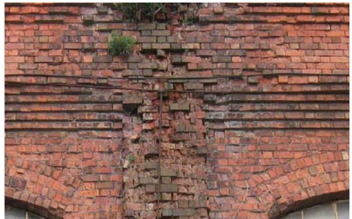
Figs 28 and 29: The site of the demolished boiler works and a typical example of neglected gutters causing severe brickwork damage
