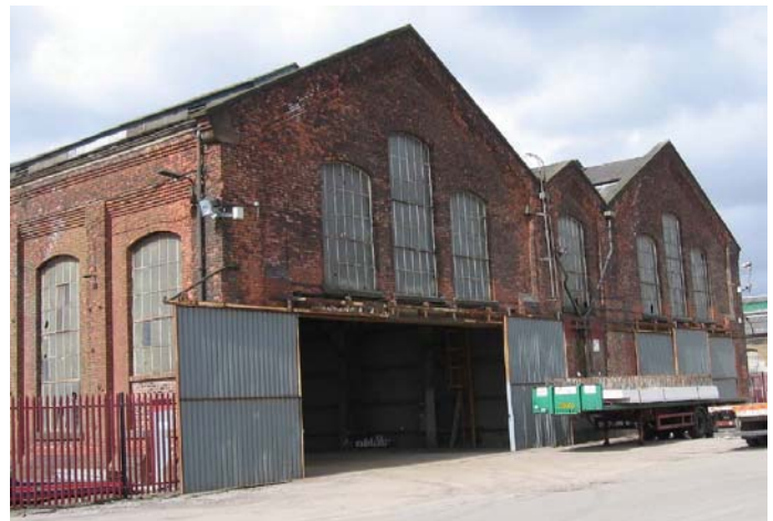
Figs 11 and 12: Part of the forge from the west left and the south west gable of erecting shop above
