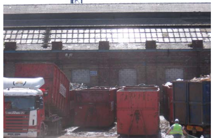
Figs 9 and 10: Fitting shop sliding door to left, spring shop chimneys visible in Fig 10
