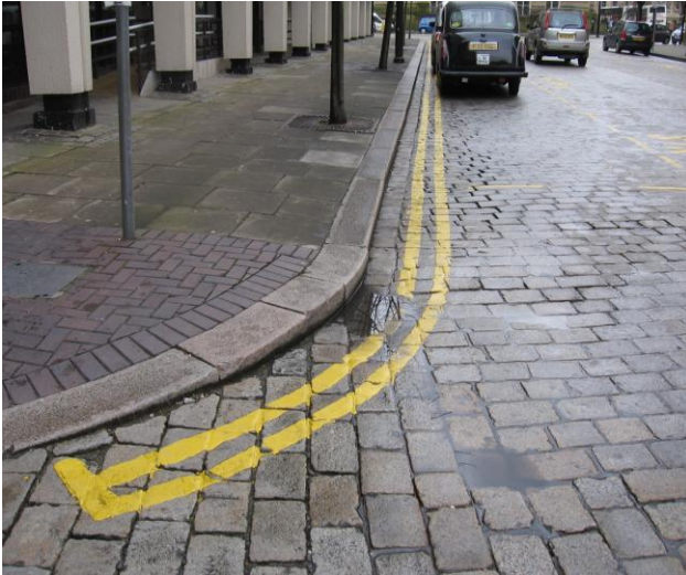
Fig.18: Granite stone setts on Howell Croft North, with stone paving and kerbs; the yellow lines are intrusive
