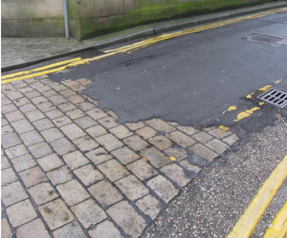
Fig.25: The tarmac laid over stone sets off the west side of Howell Croft North could be removed
