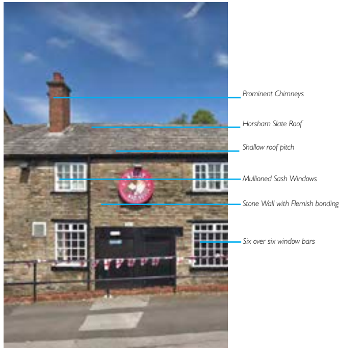
Stables House, Salford Road - an important building which displays the common characteristics of this area.
