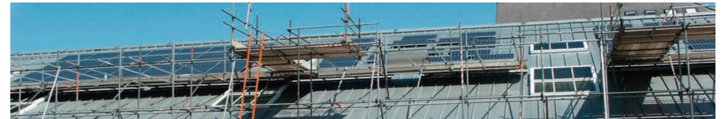
The Valley Community School photovoltaic installation
