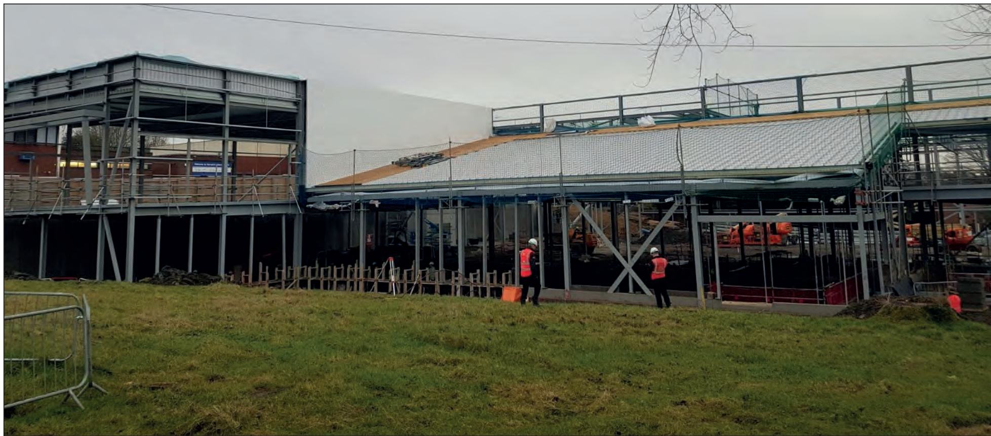
NEW BUILD: Construction on the pool at the new Horwich Leisure Centre is well underway
