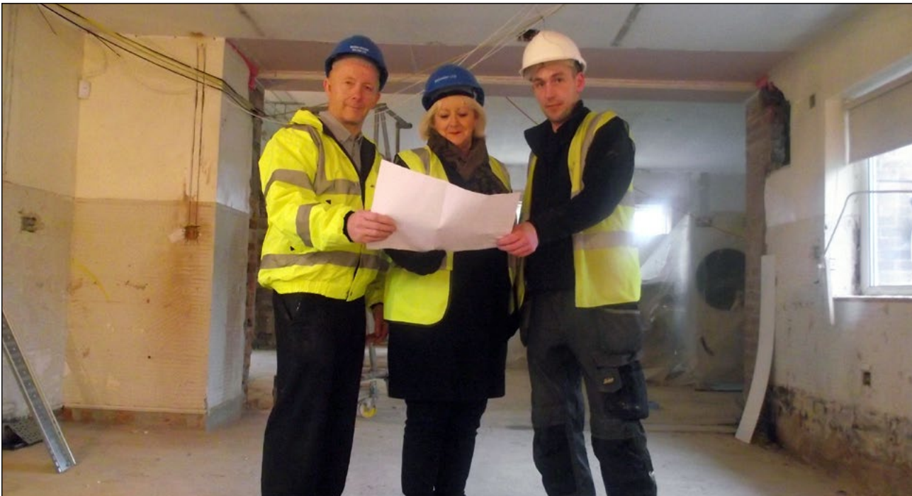
ONE CARE: Pictured (from left) are Paul Craven, MD of Medway Heating (Bolton) Ltd (left), Cllr Linda Thomas, and Darren Thomas, site manager for Medway Heating (Bolton) Ltd looking over plans in the expanded day care area
