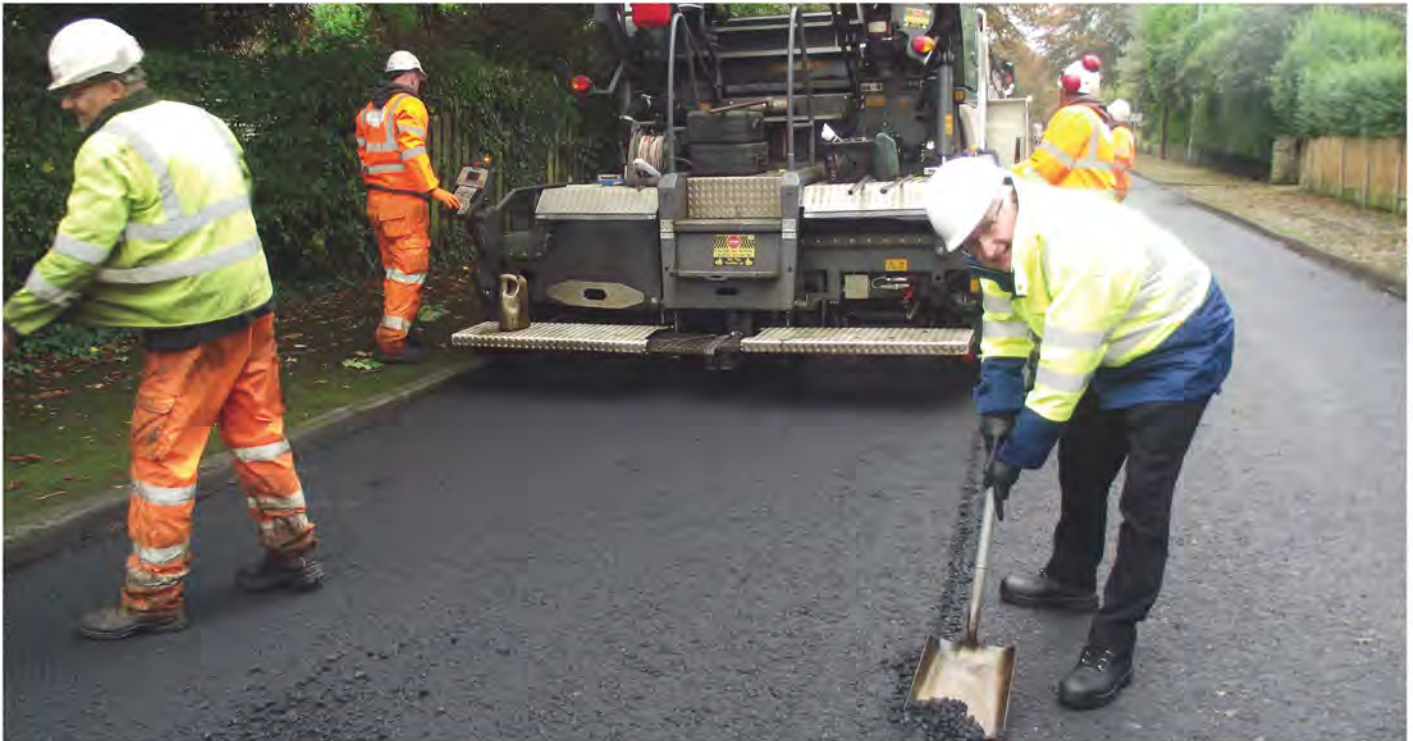
Cllr Haslam gives a helping hand to road crews at the start of the programme
